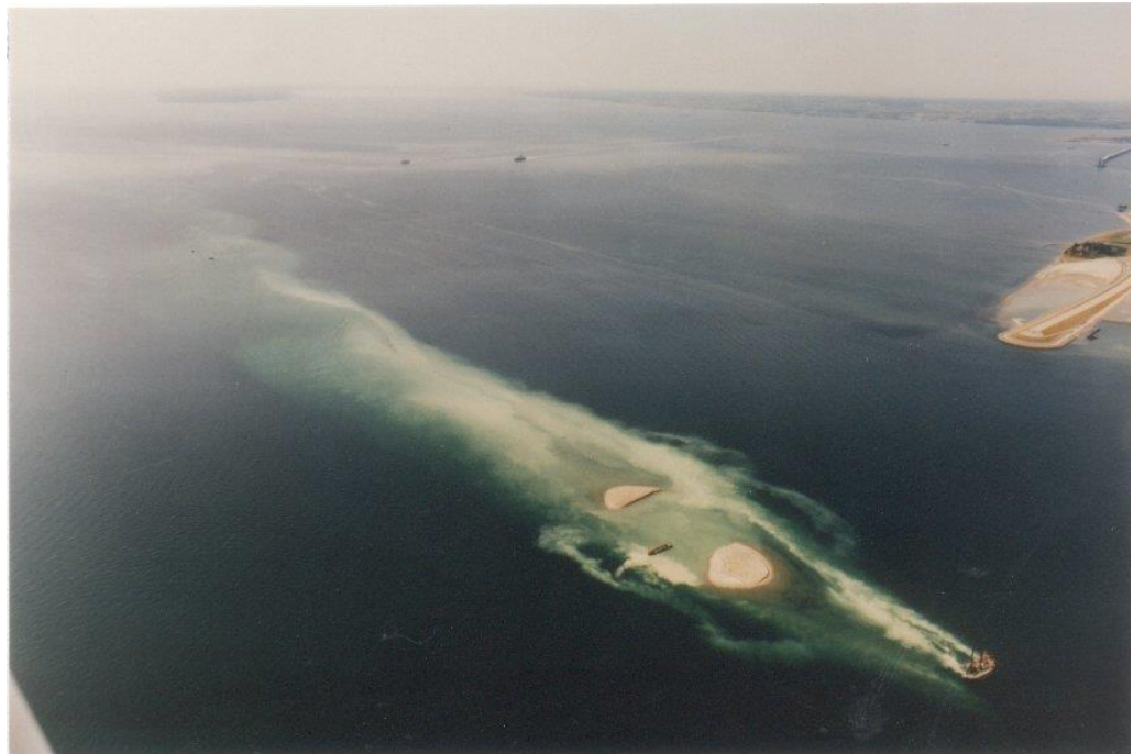
Figure 1.3 Spilled sediment during construction of pier base in the case of south-going currents. The image view is directed towards south-west
