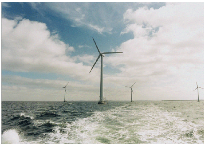
Figure 4.7 Offshore wind farm
