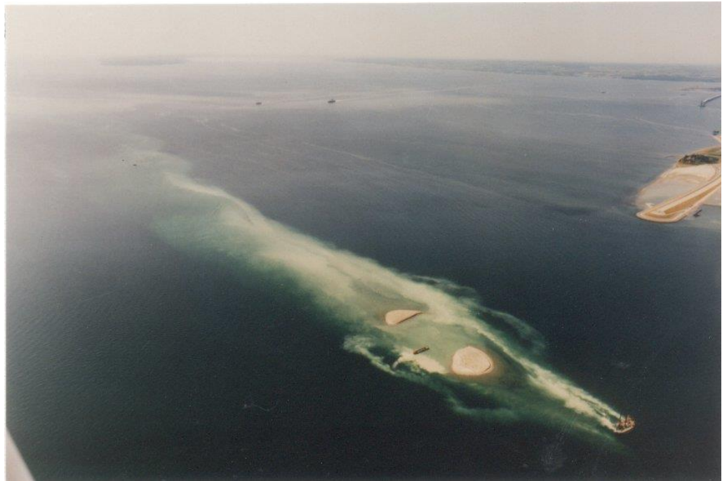
Figure 1.3 Spilled sediment during construction of pier base in the case of south-going currents. The image view is directed towards south-west
