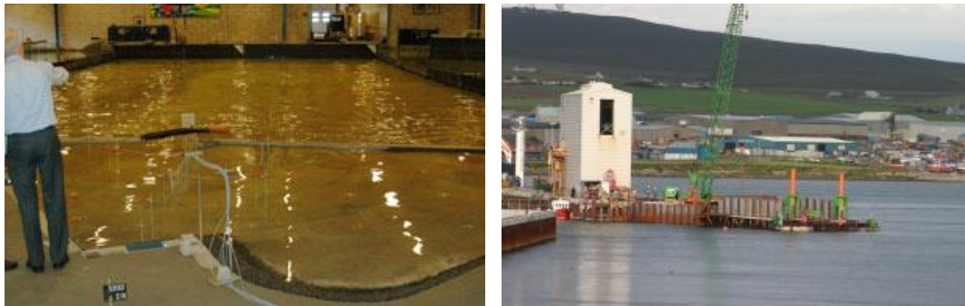
Figure 1.3 Photo of the 3D breakwater model testing at DHI (left panel) and construction of the new breakwater extension (right panel), August 2005. Images from http://www.orkneyharbours.com
